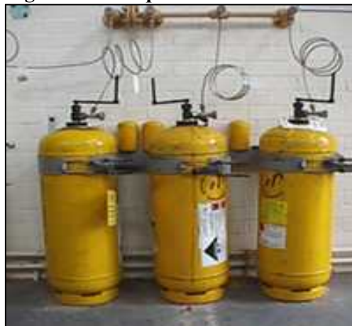
Figura 1-9 Tanque Cloro Gas
