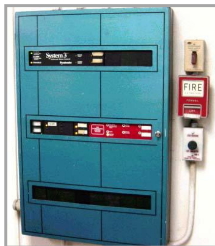
Figura 3.27 Tablero de Control
