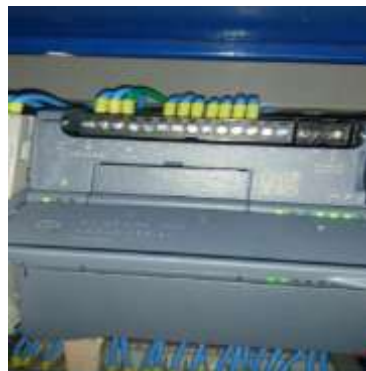
Figura 42-3: Cableado del PLC
